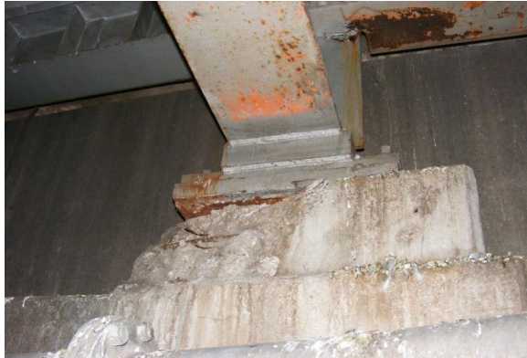
Figure 9 [Spalled Bearing Pad]
